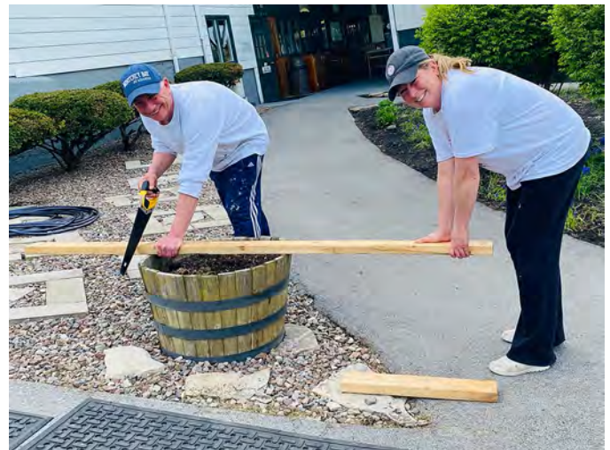
Hollie and Chris doing their good deed for the day repairing Jack Foote's bench.
